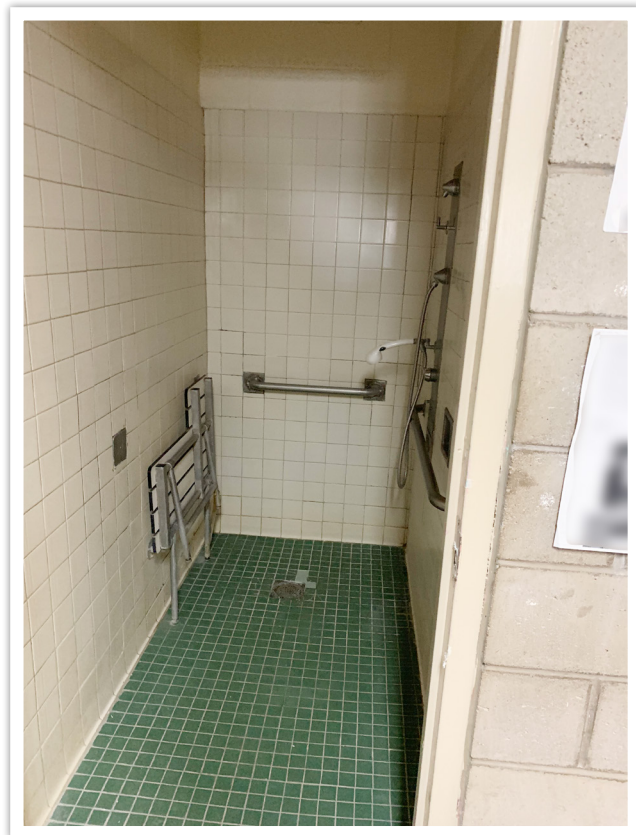
Photo 3. CCWF in-pod shower (photographed on 3-29-23).
